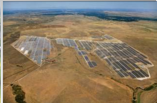
Trujillo, Extremadura, Spain-Elecnor 23 MW SunPower T0 Tracker
